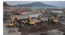
2011. Secondary screening plant Iwate Rikuzentakada-City
